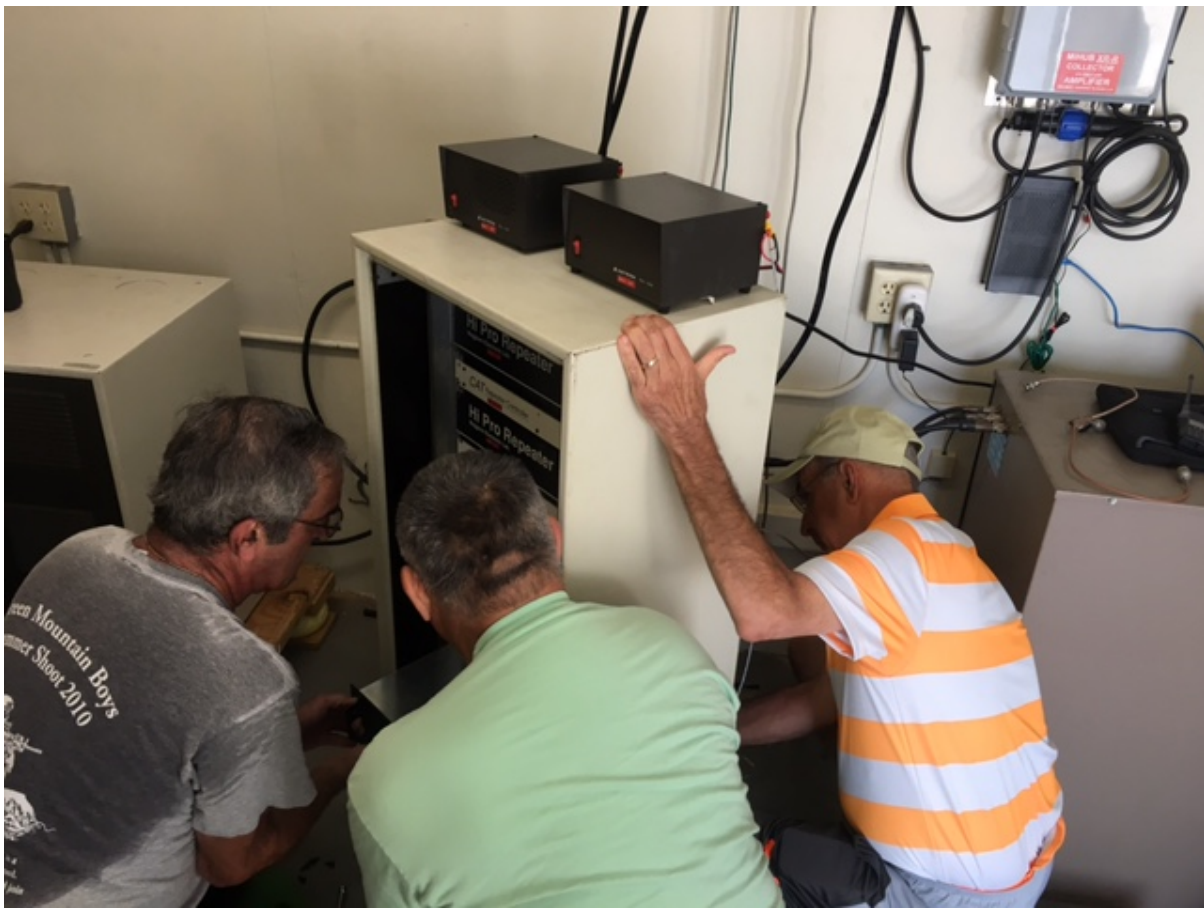
Members working Erwin Cohen-KA1DJ, Al Szoldatits- K9MDW, Tom Palmisano- W9AEB
